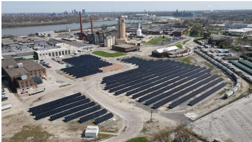
The thin film solar panels in Rossford plant
