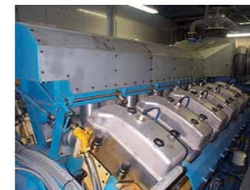
Co-generation installation, Settimo Automotive plant, Italy
