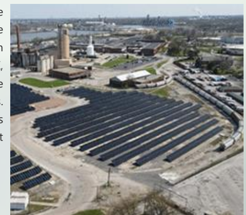
The thin film solar panels in Rossford plant
